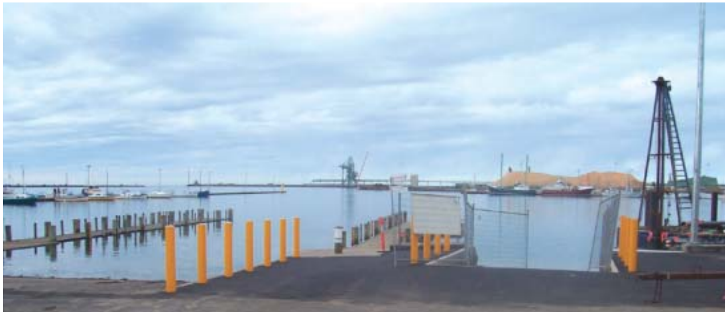
New boat lane at the Portland boat ramp, which has been constructed with funds from Marine Safety Victoria and Council , is now completed. Marine Safety Victoria's contribution of $378,200 is made possible through its Boat Safety and Facilities Program. This program is a reinvestment into recreational boating funded from a portion of recreational boat operator licensing fees and vessel registration fees.
